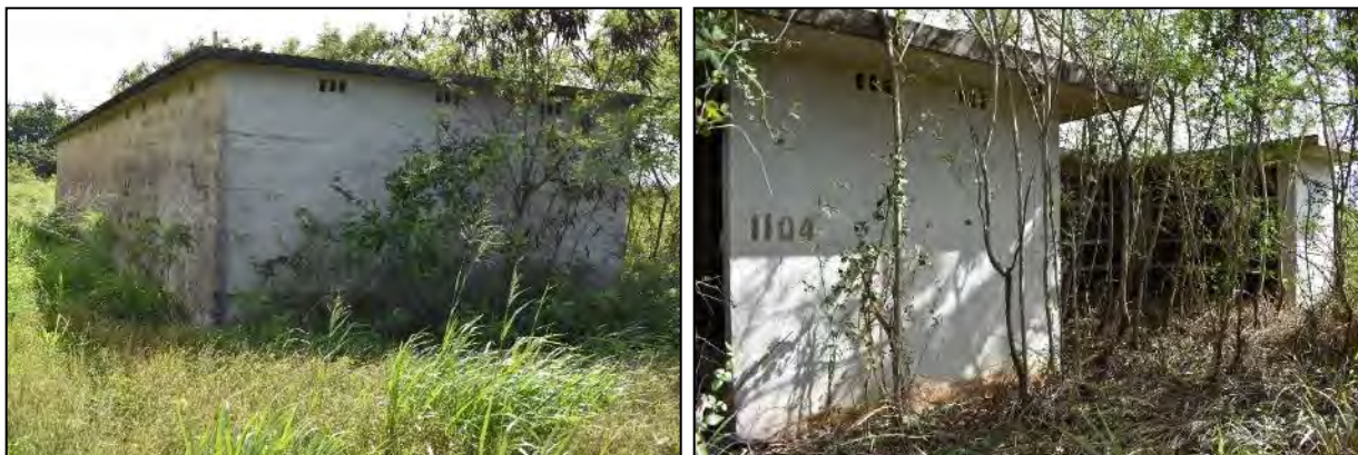
4 Building 1104 (Storage and Supply): Photo 6.1-355, left, east rear and north side elevations; Photo 6.1-356, right, west 5 front elevation
