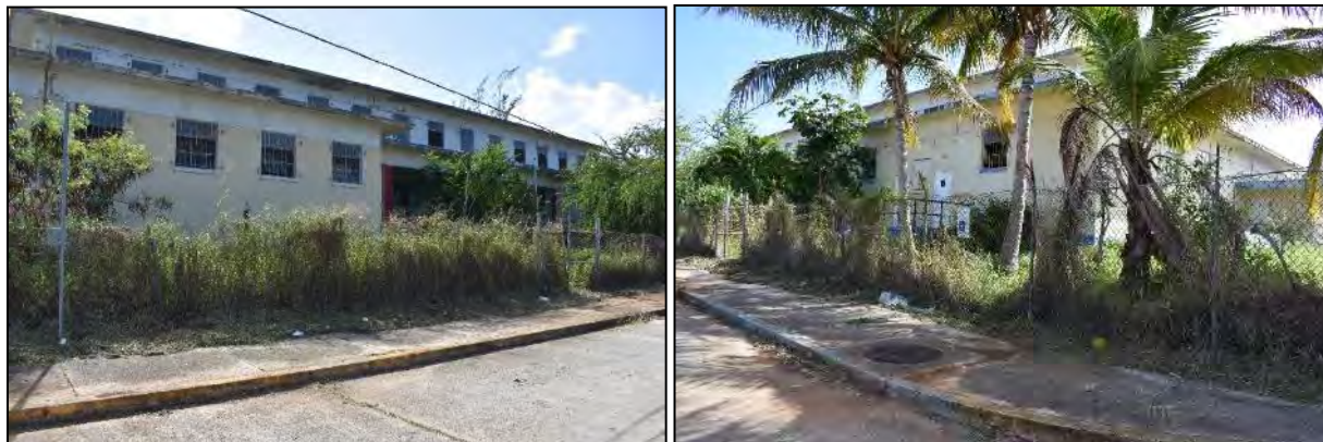
3 Building 506 (commissary): Photo 6.1-197, left, north front and west side elevations; Photo 6.1-198, right, north front 4 elevation.
