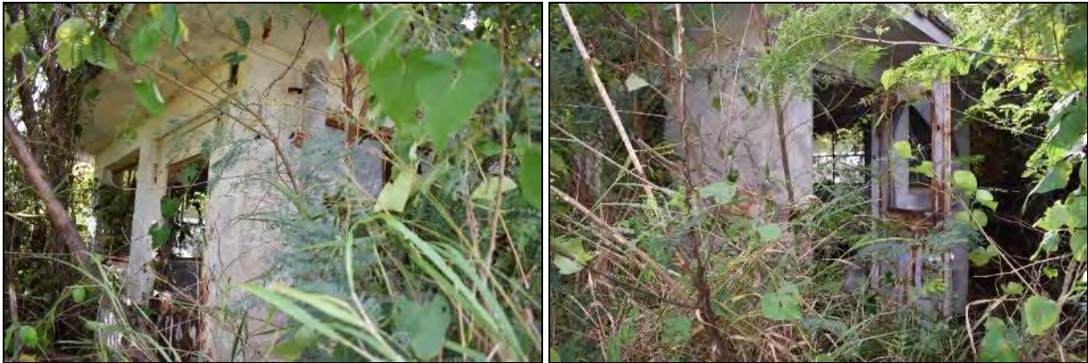
9 Building 1073 (Traffic Check House): Photo 6.1-419, left, south front and east side elevations; right, east side and north 10 rear elevations.
