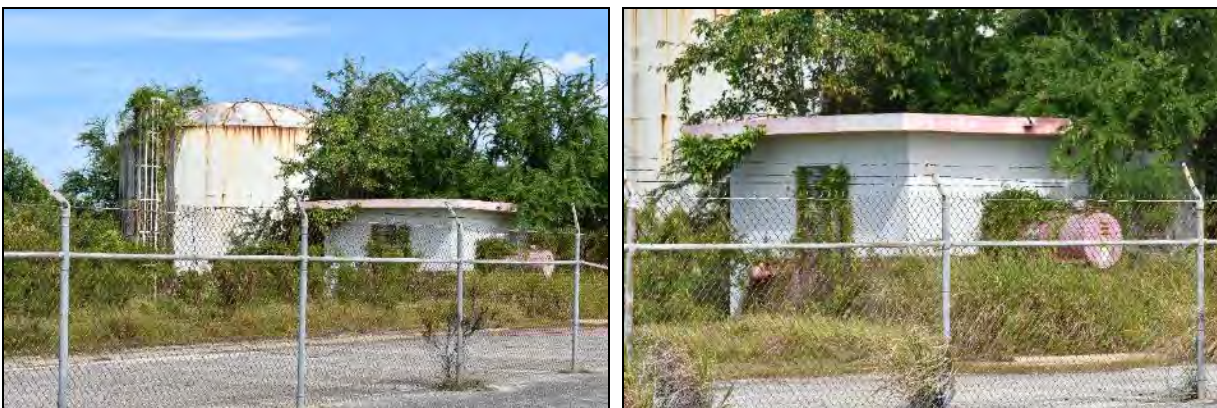
13 Electrical Station: Photo 6.1-389, left, east and south elevations with water tank looming to rear; Photo 6.1-390, right, 14 east and south elevations
