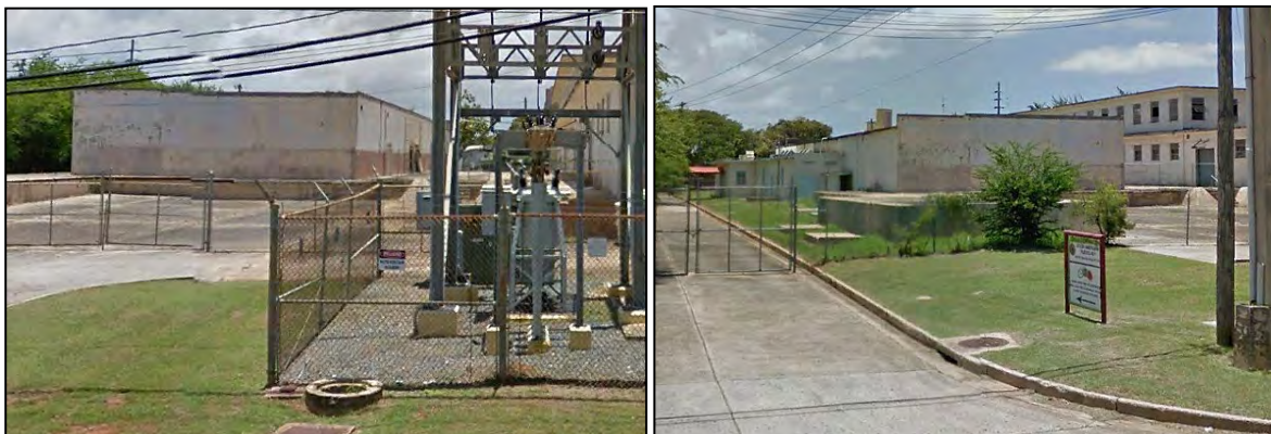
3 Building 509 (Cold Storage Plant): Photo 6.1-208, left, north front and east side elevations; Photo 6.1-209, right, east 4 side and south rear elevations (source: Google Earth, dated May 2016).
