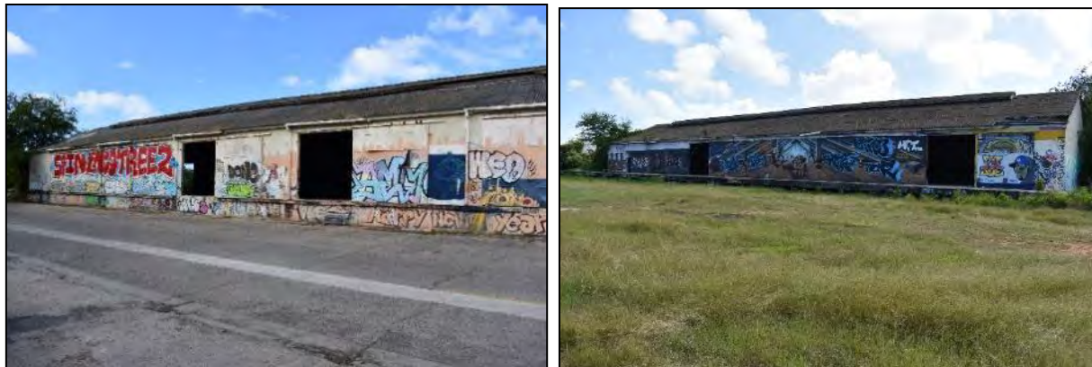
1 Building 512 (Quartermaster Warehouse): Photo 6.1-216, left, north track-facing and west side elevations; Photo 6.1- 2 217, right, south road-facing elevation.
