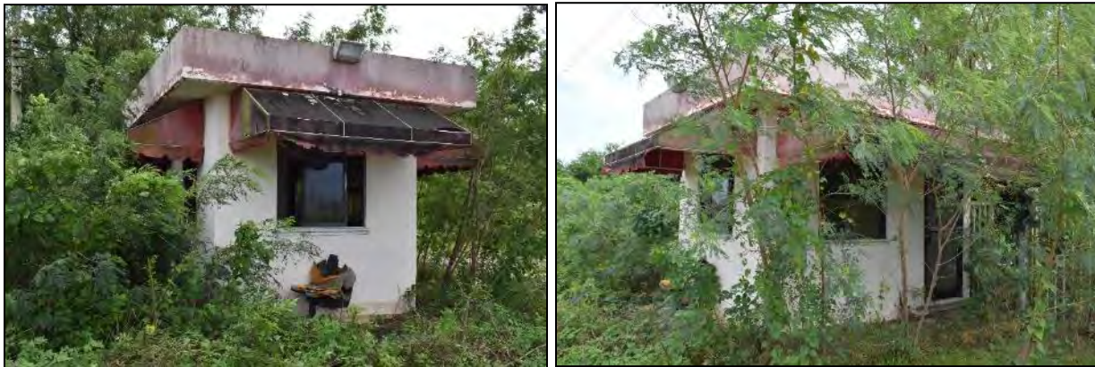
9 Guard House: Photo 6.1-362, left, west side and south front elevations; Photo 6.1-363, right, south front and east side 10 elevations
