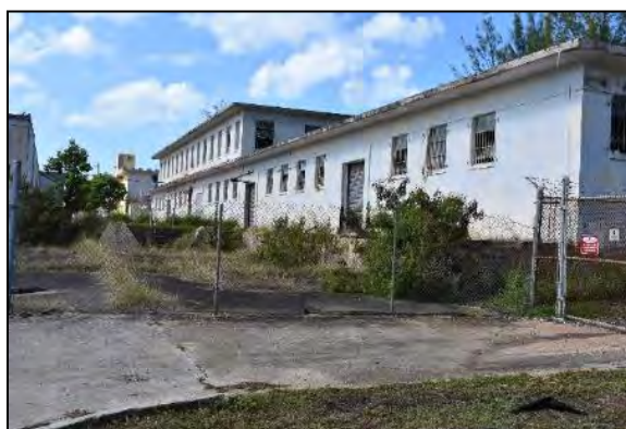
5 Photo 6.1-210, Building 509 (Cold Storage Plant): northeast corner of building at far left with rear of Building 508 in 6 front.
