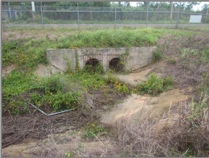
These images show part of the stormwater system (ditches and inlets) at the airport.
